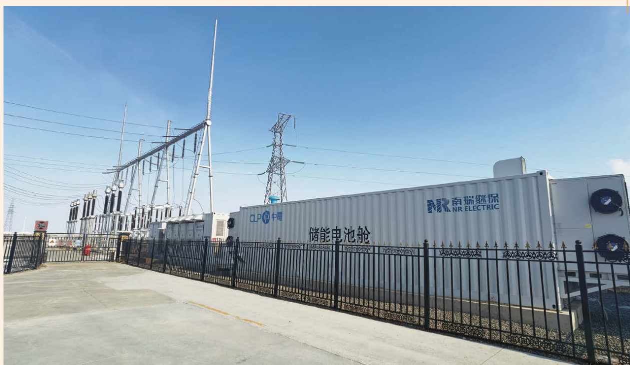
Qian'an III Wind Farm in Mainland China is the first CLP project of its kind equipped with a battery energy storage system.
