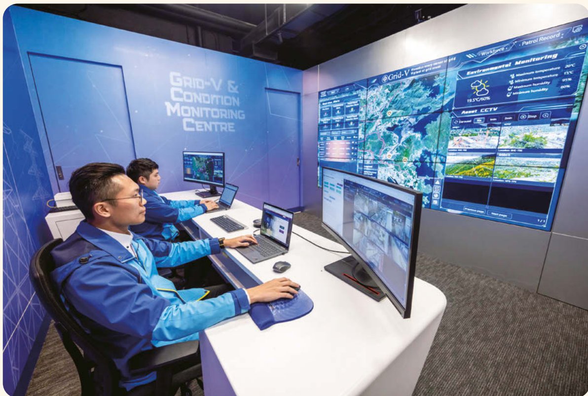
■ CLP Power's Grid-V system uses AI-assisted analysis to enhance the monitoring of the power grid.
