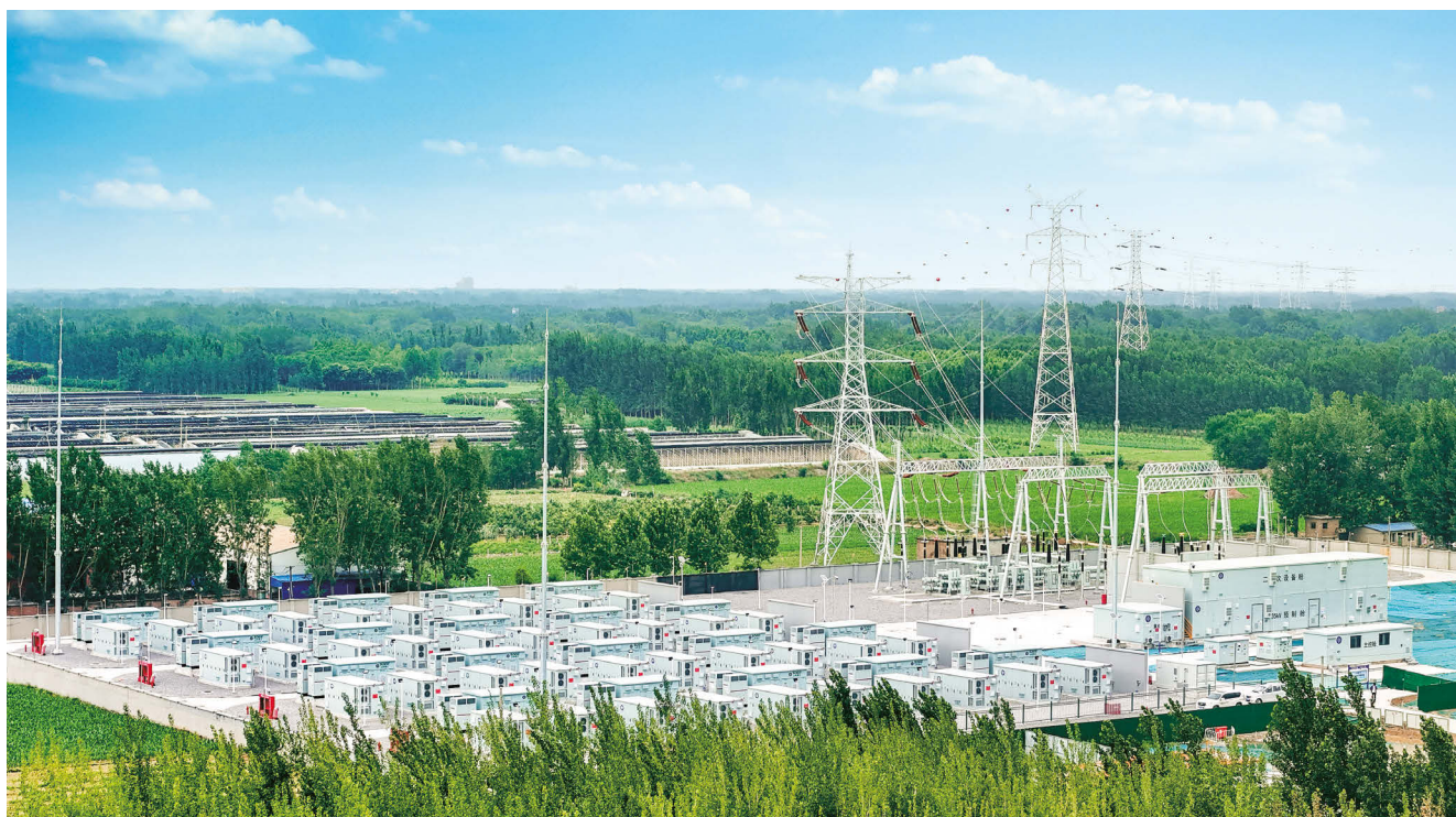
Commissioned in 2025, the Guanxian Battery Energy Storage System in Shandong province is CLP China's first independent BESS project.
