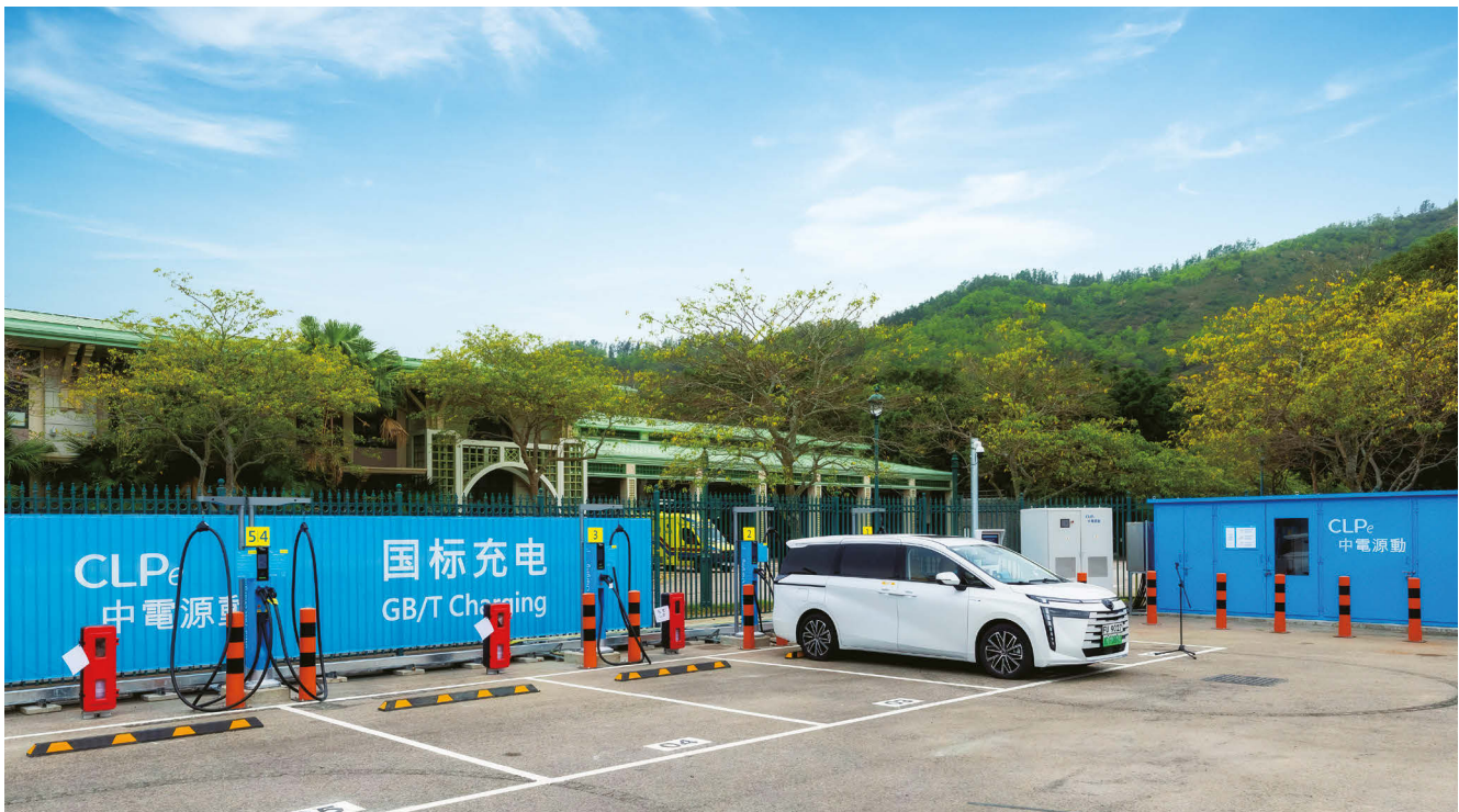
CLPe supports the Government's Southbound Travel for Guangdong Vehicles Initiative with a new EV charging station on Lantau Island.
