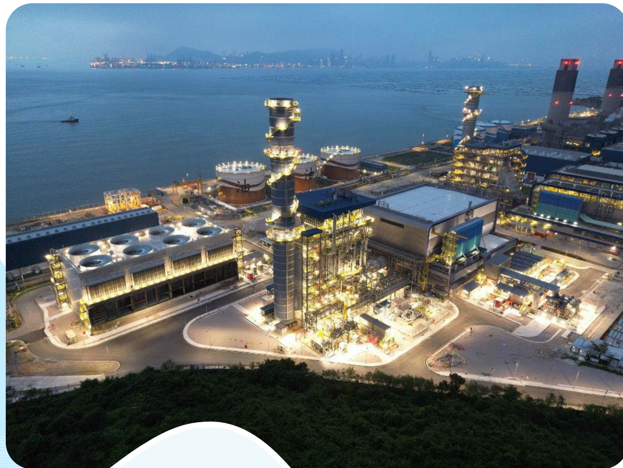
CCGT D2 gas-fired generation unit at Black Point Power Station, Hong Kong.
