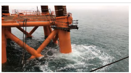
Use of bubble curtain as mitigation measure to further reduce underwater noise from piling during jetty construction
