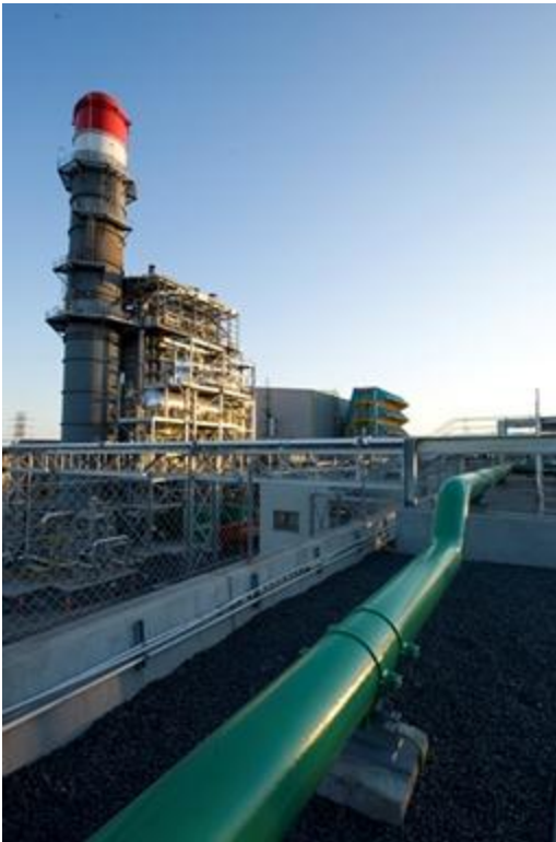
TRUenergy Tallawarra 435MW Gas-fired Power Station
