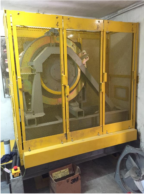
The lift at Cheung Hing House in Mongkok after energy efficiency improvement works subsidised by the CLP Eco Building Fund.
