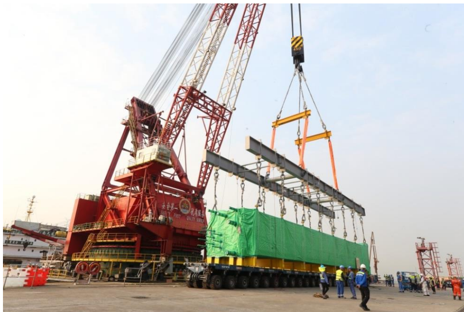
One of 15 Heat Recovery Steam Generator heat surface modules is unloaded. Each is more than 30 metres long – equivalent to the length of three double-decker buses.
