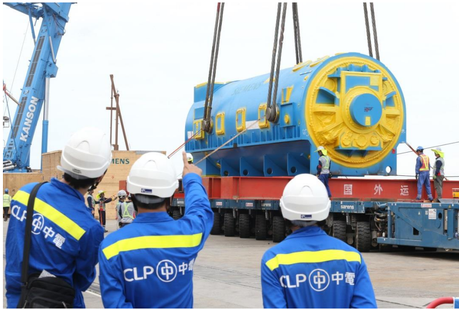
The generator for the gas-fired generation unit, also weighing around 450 tonnes, is unloaded.
