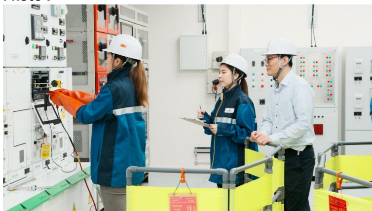
The High Voltage Training Centre in the new Lab enables learners to take high voltage training programmes accredited by the Electrical and Mechanical Services Department, helping them gain the Grade H Registered Electrical Worker qualification.
