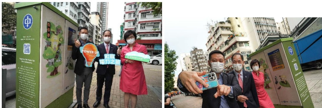
(From left) Secretary for Home Affairs Mr Caspar Tsui, Managing Director of CLP Power Mr T K Chiang and Chief Corporate Development Officer of CLP Power Ms Quince Chong visited a beautified distribution box in Sham Shui Po after the launch ceremony for the Distribution Box Beautification Project , titled “Together We Power Up Our Community” .
