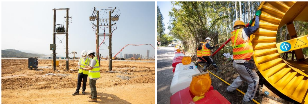
CLP Power engineering team and contractor staff lay 8 kilometres of cables to the Lok Ma Chau Loop in a record 10 days.
