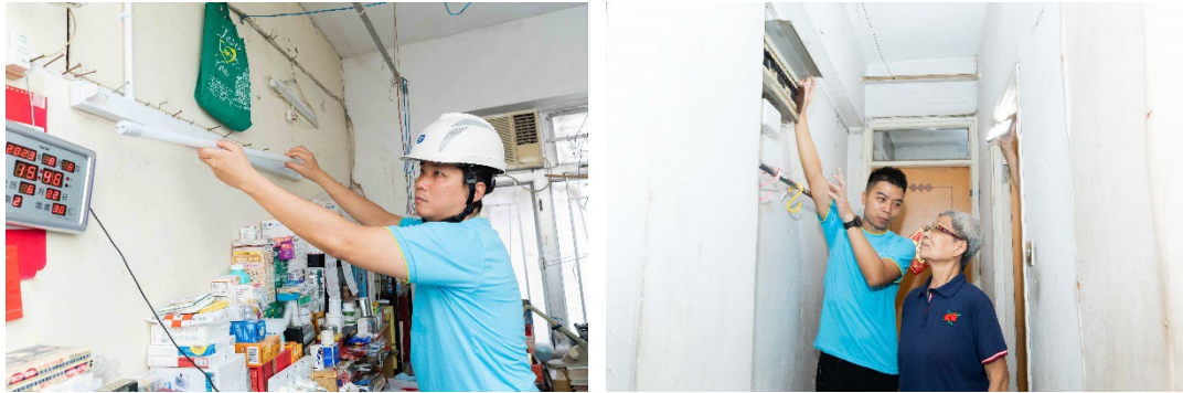
CLP volunteers install fluorescent light and inspect the electrical distribution board in Ms Lam's apartment.
