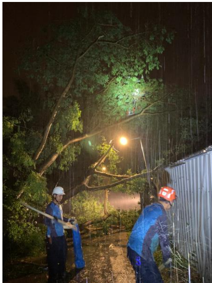
CLP Power's engineering team has been on duty to safeguard reliable power supply during the typhoon.
