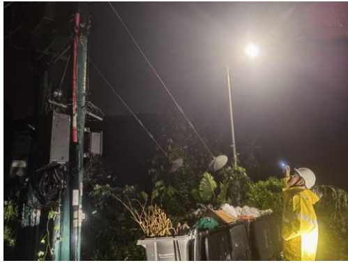
CLP Power's engineering team is carrying out inspections of the power supply equipment during Super Typhoon Saola.
