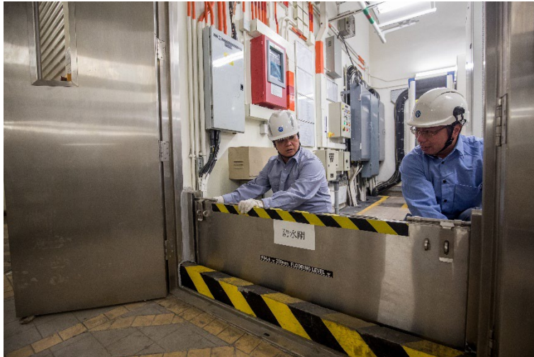
CLP Power installs flood gates at flood-prone substations to mitigate flood risk.
