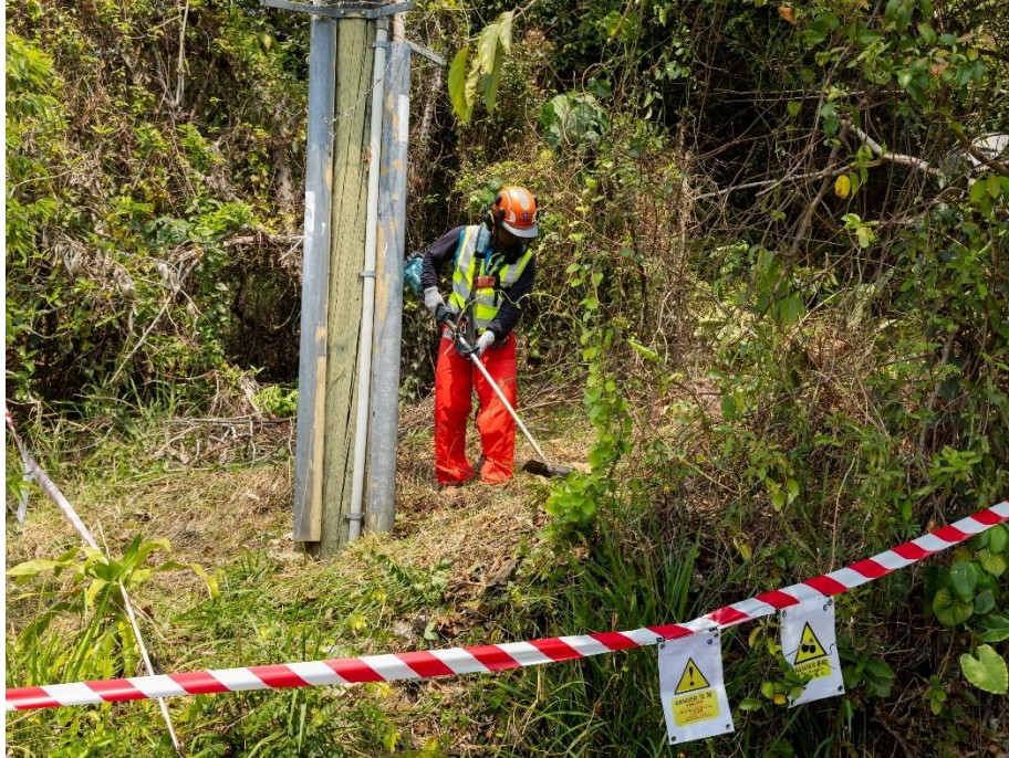
CLP Power conducts pole cleaning at over 400 locations to remove nearby weeds and tree branches, minimising potential impact of hill fires on power facilities.
