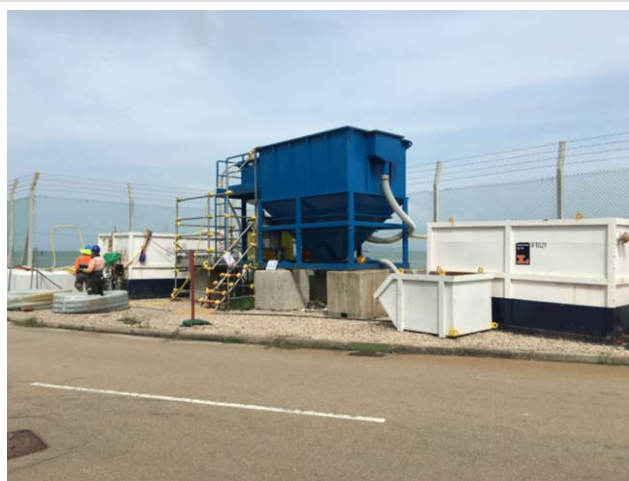
Site waste water treated with desilting and water treatment plant before discharge
