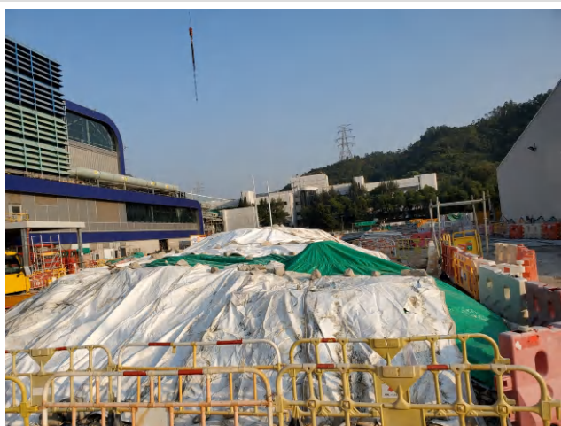
Cover stockpile of soil material to prevent generation of fugitive dust and surface run off
